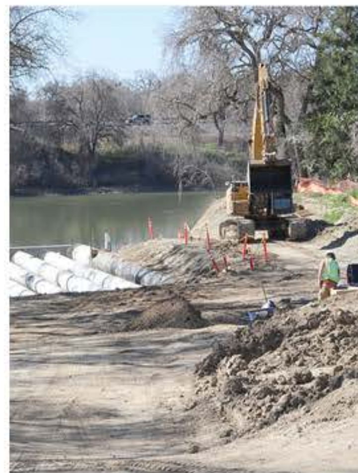
Pump 4 repair on Garden Highway above San Juan Road directly on the river.
